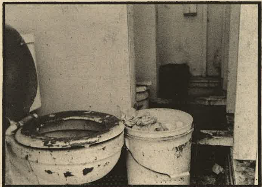
These are flush toilets. At the time we visited they did not work. There are safety hazards of 2 by 4's up from and across the floor.
